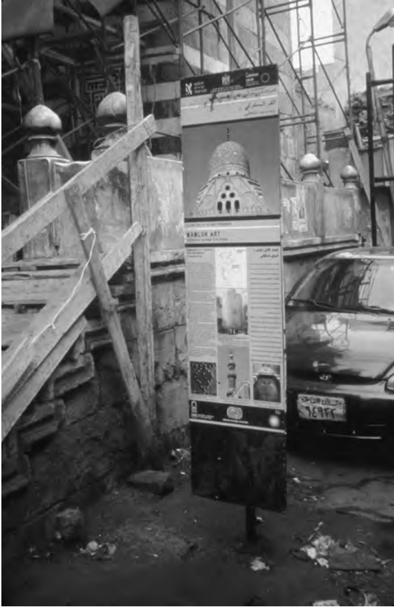
The "Museum with No Frontiers" sign sits in place although the complex of Sultan Barsbay and other buildings around it are still being reconstructed (photograph by Caroline Williams).
