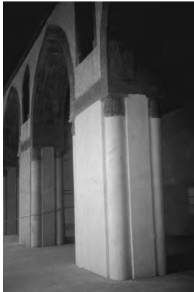
Mosque of Ibn Tulun, side arcade. Pier, on left, covered with new plaster undercoat; pier, on right, covered with final coat of twentieth-century stucco (photograph by Caroline Williams).
