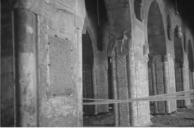
Mosque of Ibn Tulun, sanctuary arcade. Pier, on left, with original stucco and ninth-century foundation tablet. Piers, behind yellow tape, showing bare brick after removal of stucco (photograph by Caroline Williams).
