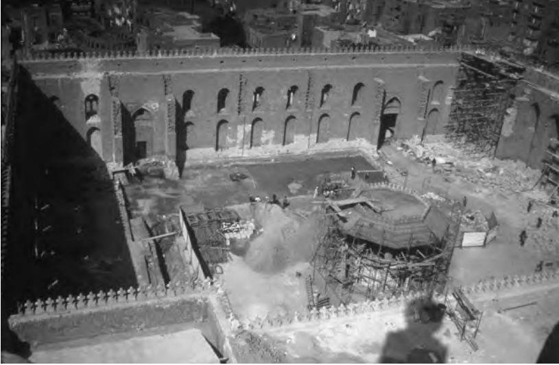
Looking down into the interior courtyard of the mosque of al-Muayyad Shaykh where the Wadi al-Nil Construction Co. is completely reconstructing the courtyard and side colonnades (photograph by Caroline Williams).
