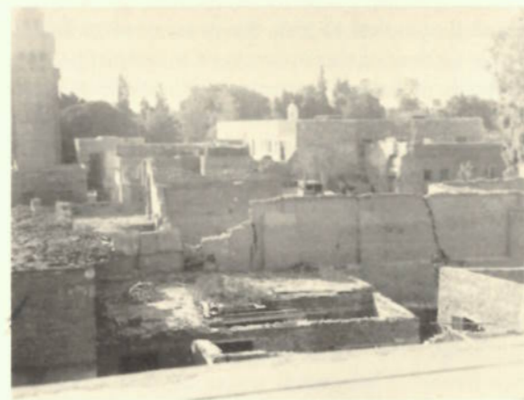
129. Old homes crumble. A roof view in the walled compound of Miṣr al-Qadīmah
