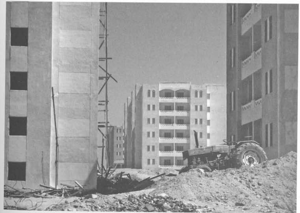
Figure 5.9. New National Housing Program public housing block under construction, Sixth of October, 2009. (Photograph by Sonja Spruit.)
