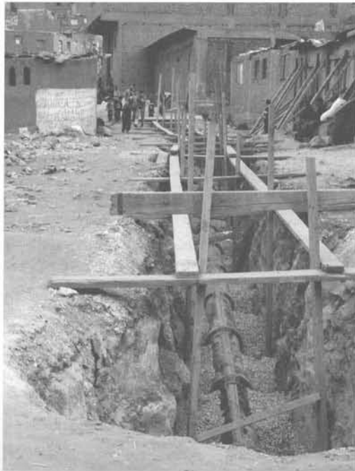
Figure 9.1. Installation of water main by government to serve informal areas of Manshiyat Nasir, 2002. (Photograph by David Sims.)
