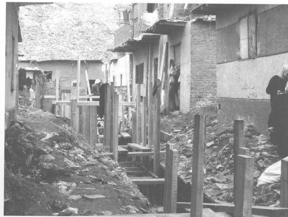
Figure 9.2. Installation of local sewers and house connections: project financed by German Financial Cooperation, in 'Izbit Bikhit (Manshiyat Nasir), 2001. (Photograph by David Sims.)
