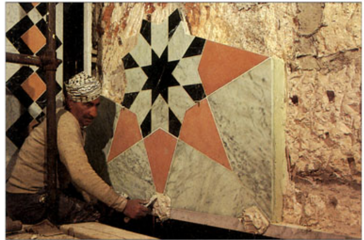
Opposite: Other restoration and re-use programmes in the area include the Fakhriyya Minaret and Islamic Museum (top) and the Sabil of Qaytbay (with scaffolding) in the western courtyard (bottom). Above: Installing marble wallfacings.
