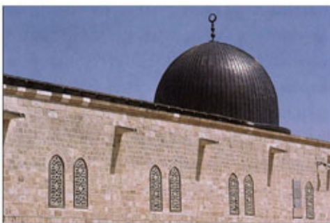
Al-Aqsa Mosque, Jerusalem: technically outstanding restoration work carried out under exceptionally difficult circumstances.
