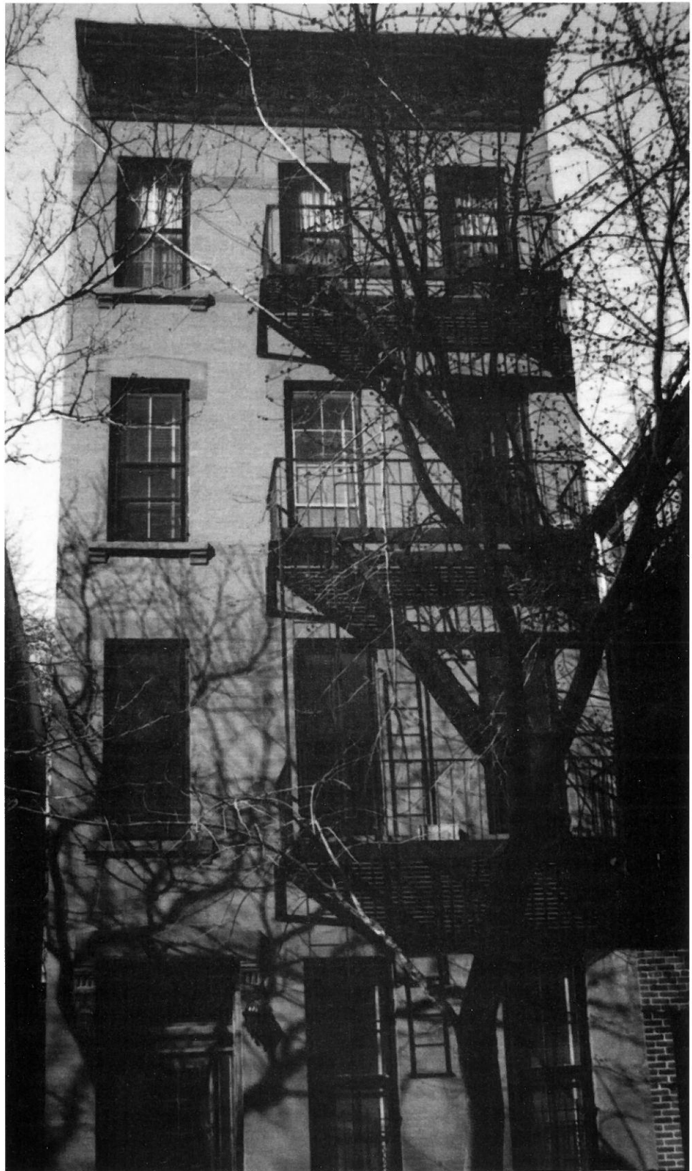
Dumbbell, elevation. The fire escape, mandated by law in 1867, reveals a working-class dwelling despite decorative allusions to the middle-class row house
